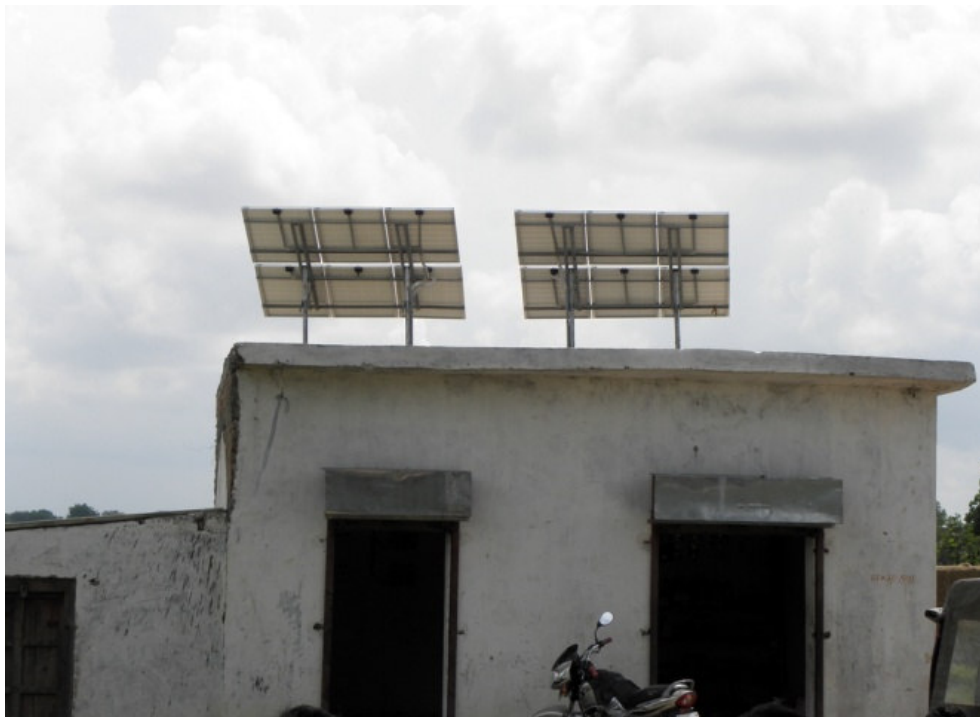
Picture 2. Solar Charging stations in Kacchuwa (Outside)
