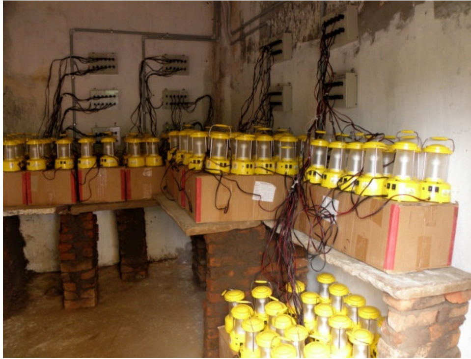
Picture 1. Solar Charging stations in Kacchuwa (Inside)
